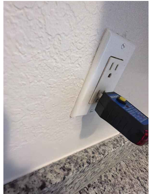
Cannot plug in bottom outlet, kitchen above DW
